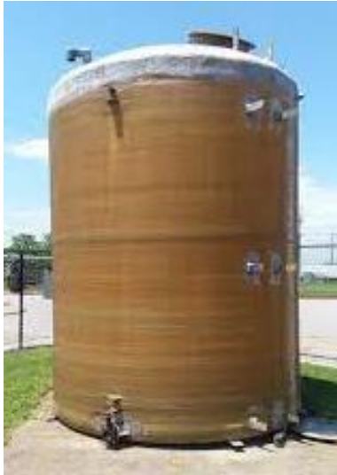
Fiberglass Water Tank
